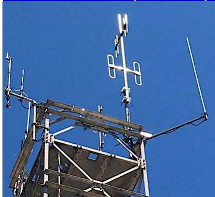
photo shows the new quad dipole TX antenna
